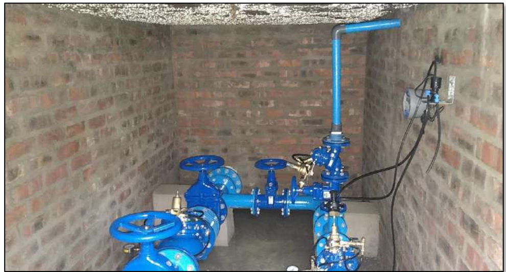
View of the PRV Configuration with 2-step Controller and Solenoid Valve
