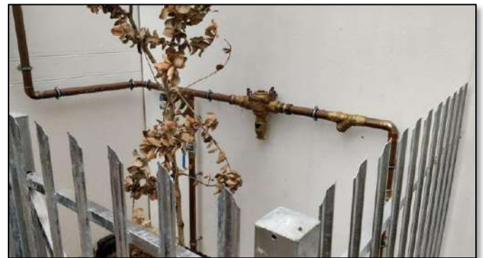
RPZ Valve Installations
