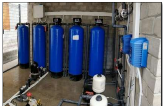
Water Treatment Works
