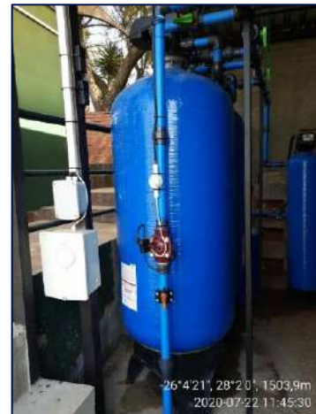
The solenoid valve and electrical cabling for plant automation
