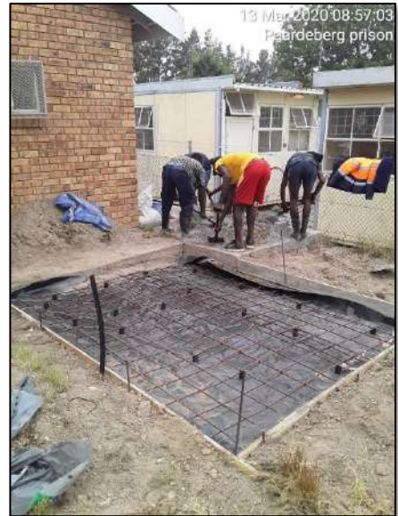
Excavation and reinforcement for the 200mm concrete slab to house the WTW
