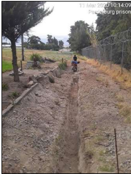
Excavation for the raw water pipeline from the borehole to the Water Treatment Works (WTW)
